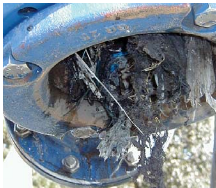
Solids and fibres can cause serious problems.
