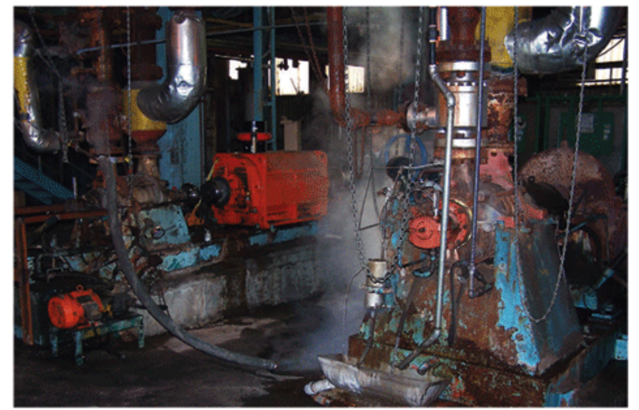
Pumps on location in Castlegar, BC. The HDA pump on left has electric motor drive while the one on right is driven by steam turbine. Left: Sectional drawing of the pump type used at Celgar.
