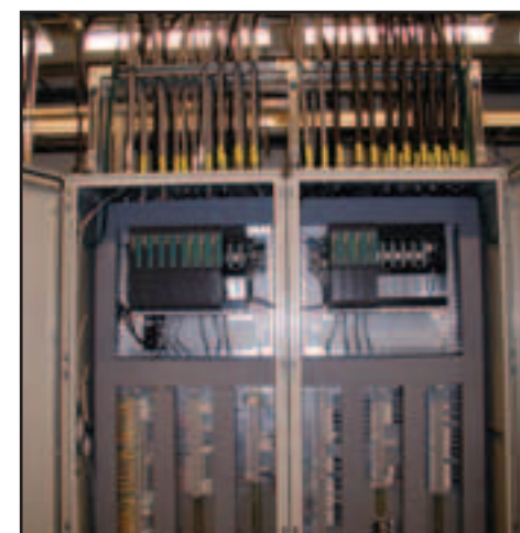
TS8 enclosure for Fossil boiler management system.
